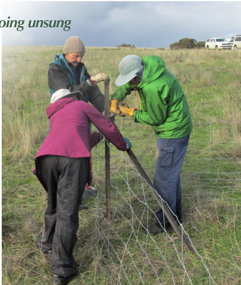
Building an enclosure at Dananbilla Nature Reserve, NSW. Photo by Brian Slee
